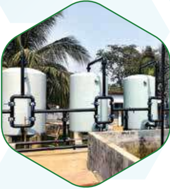
Iron Removal Plant
