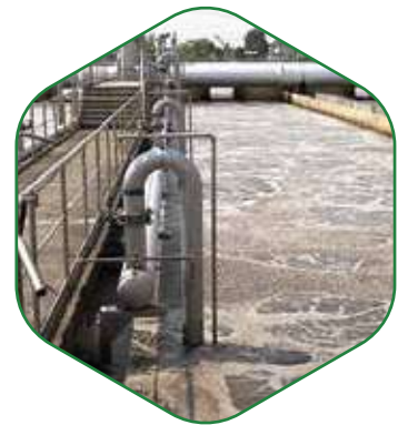
Sewage Treatment Plant (STP)
