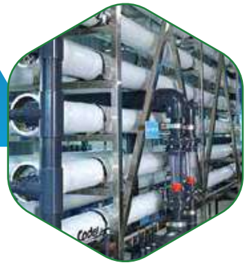
Membrane-Based Desalination Water Treatment Plant
