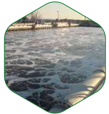
Waste Water Recycling Plant
