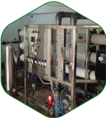
RO Water Treatment Plant
