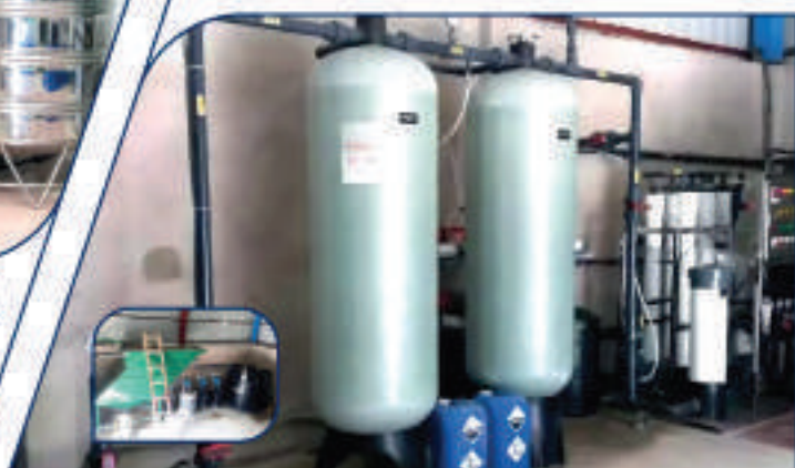
Lake Water Treatment Plant Client: Golden spot Limited, Shikunda, Chittagong Capacity: 02 m 3 /hr RO & 05 m 3 /hr Pre-treatment system
